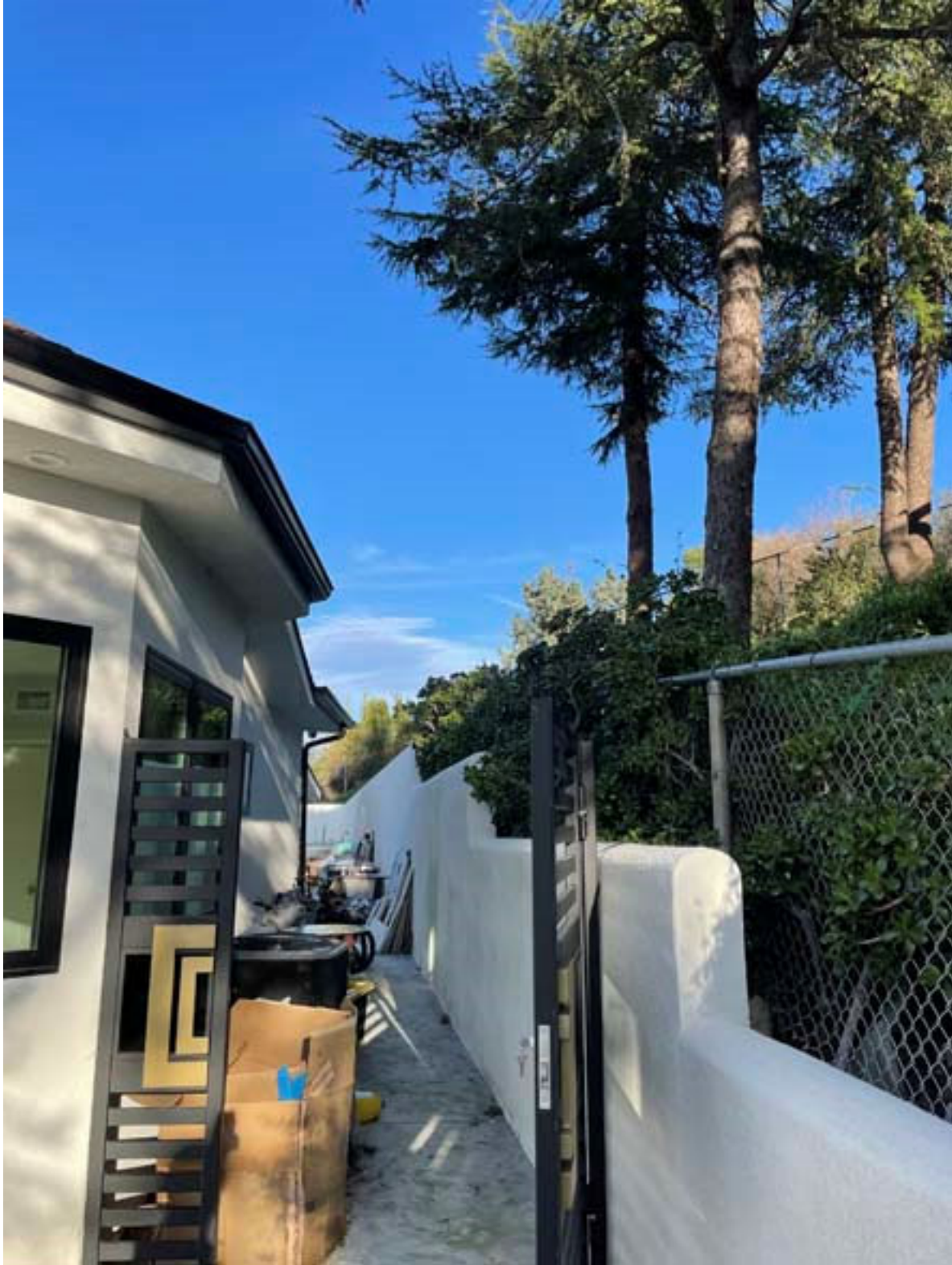
Figure 24: Looking east along the southern property line. A retaining wall separates Trees OP17, OP18, and OP19 from the area where construction work occurred.
